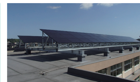
Rooftop solar power station installed on a public facility
