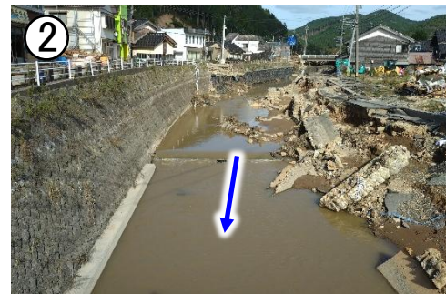
護岸の被災状況(鈴屋川)
